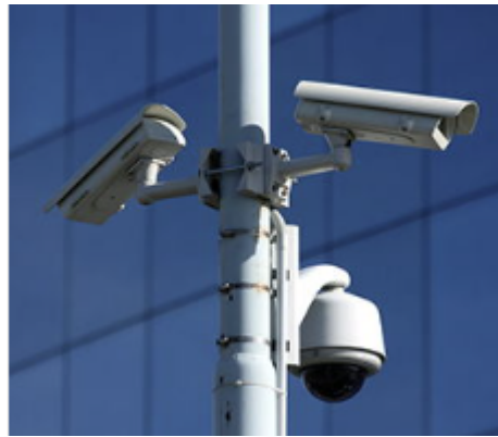
Figure 8. Video Camera Installation
